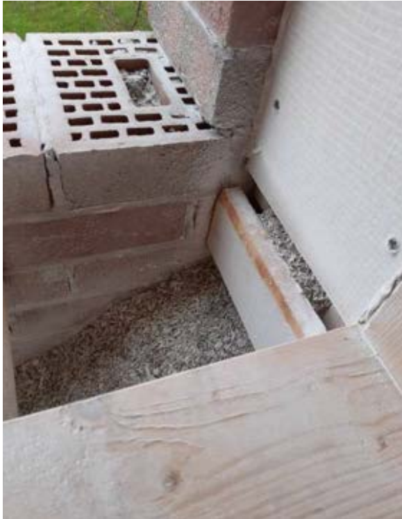
BLAF architecten, jtB House.
