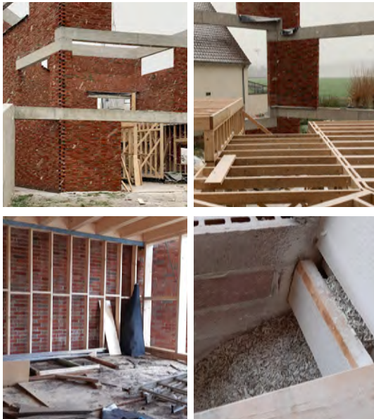
The construction of the jtB house Brick shell and timber frame, limehemp insulation with no ventilated cavity (right)
